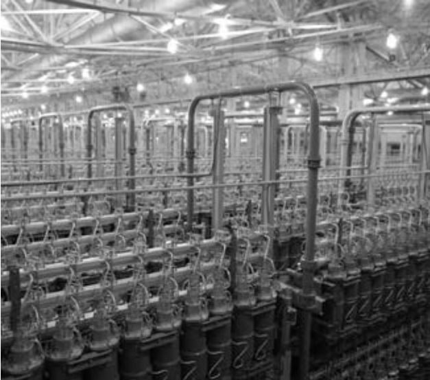
Centrifuge facility at the JSC "UEIP" ↑
